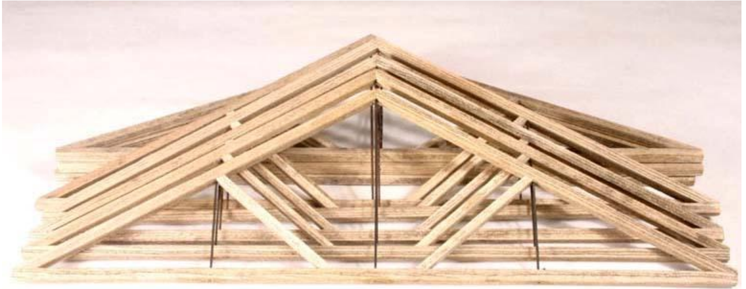
Trusses for the “New Mill”. More trusses were made than indicated in the SierraWest Twin Mills at Deer Creek to accommodate the custom larger mill. Note the vertical steel rods which were installed using the tool mentioned above.
